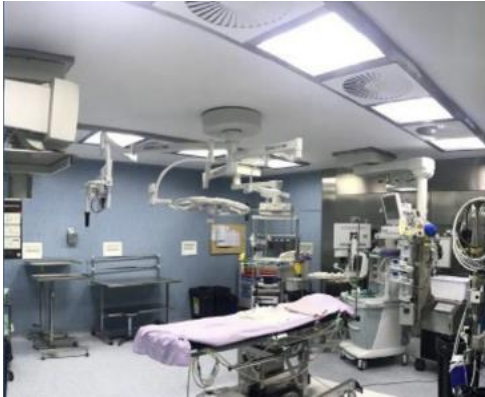
Montevergine Hospital – Operating Room – Department of Cardiology Campania
